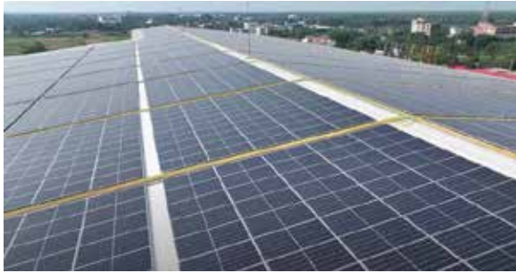
Image of 2.2 MW capacity Solar Panel Installation.
