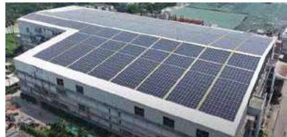
Image of 2.2 MW capacity Solar Panel Installation
